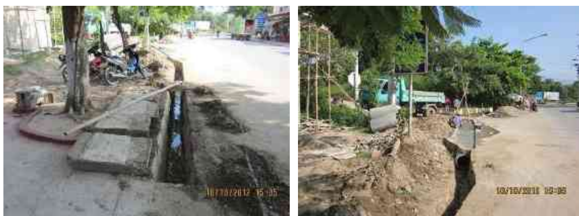
Figure 21. Left: Cleaning activities of Drainage channel by the Luang Prabang Province - Urban Development and Administration Authority (UDAA), Right: Picture of Drainage repair works by UDAA (UDAA 2013)
