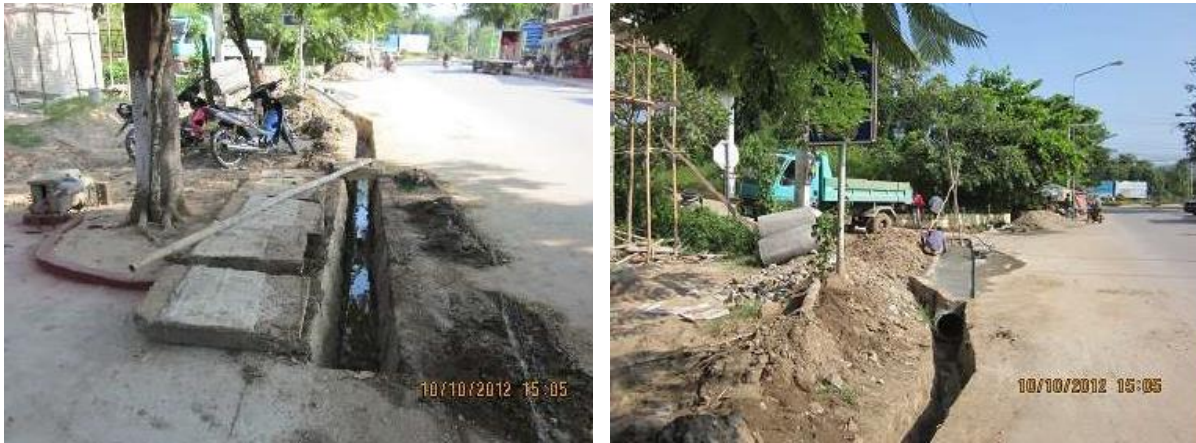
Figure 5. Left: Cleaning activities of Drainage channel by UDAA, Right: Picture of Drainage repair works by UDAA (sourced from the Luang Prabang Drainage and Sewerage System Master Plan, 2023)
