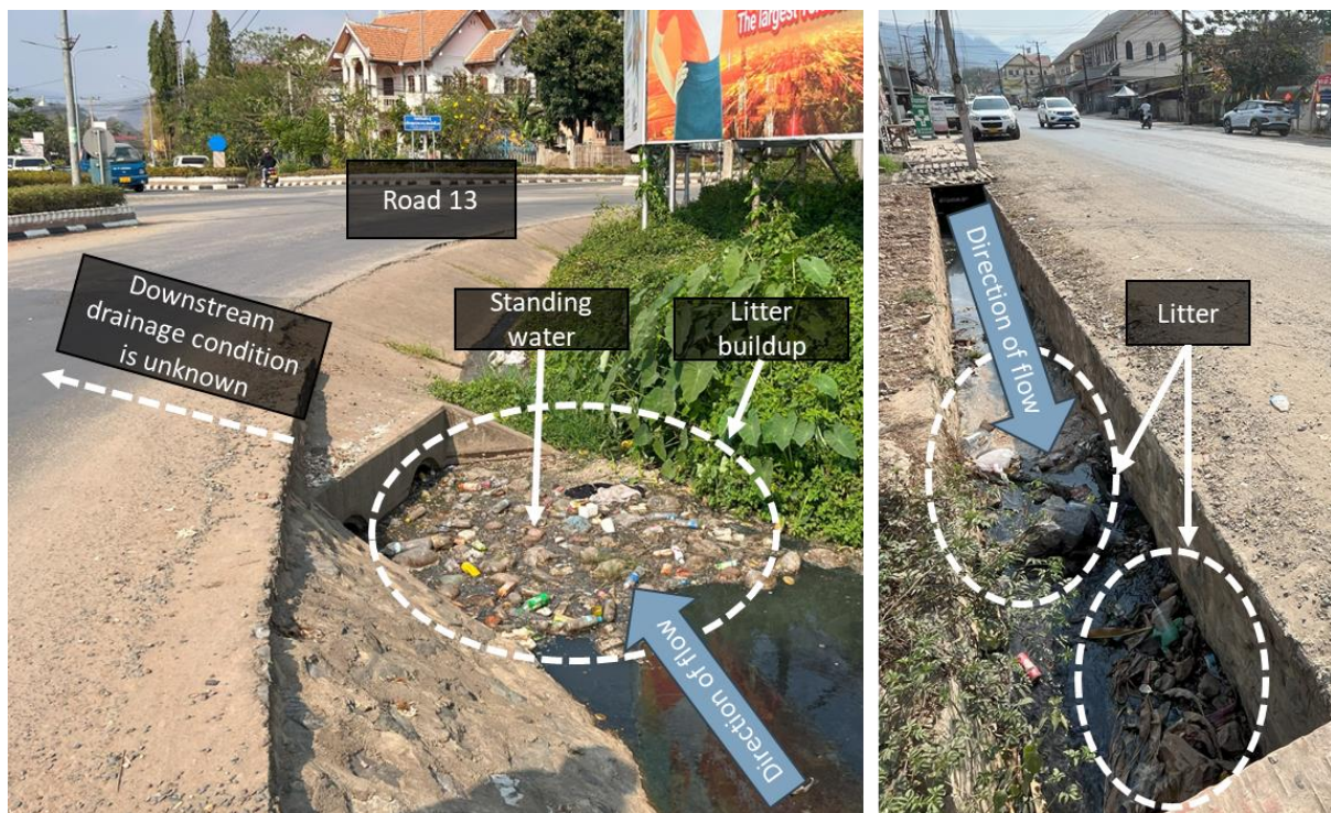
Figure 23. Left: Road 13 corner junction (facing downstream). Right: Road 13 corner junction (facing upstream)
